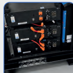
FULLY SELF-CONTAINED LiFePo 4 lithium batteries
